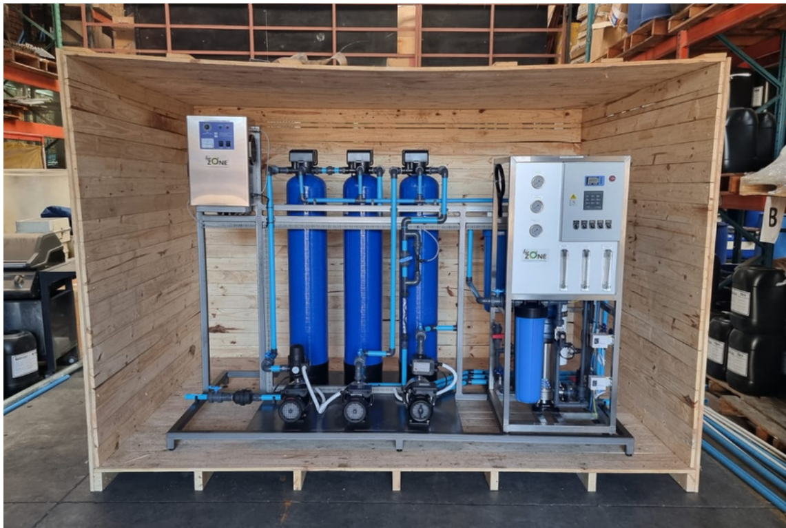
Off grid Water Purification system and purified bottled water solution in Botswana. 1000 litres per hour Water Treatment Plant including bottling equipment directly from a borehole in Francistown Botswana.
